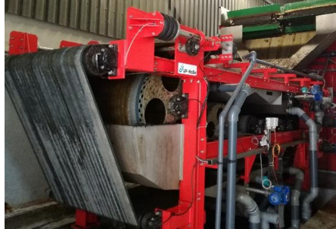
Belt press. Source: VP-Hobe, installed at BioStorg Biogas Plant, Houthalen-Helchteren, Belgium, 2019.
