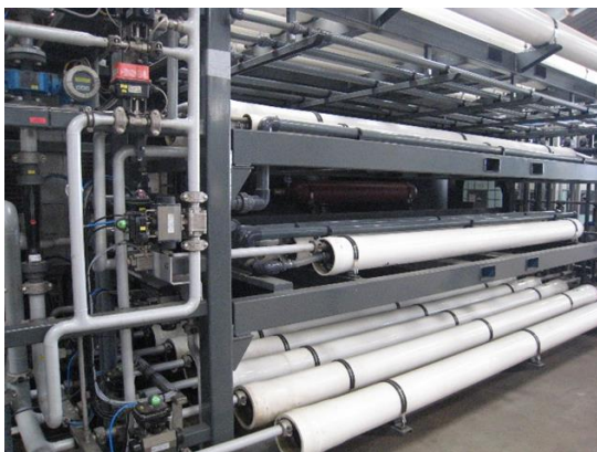
Photo 1. A Reverse Osmosis (RO) installation.
